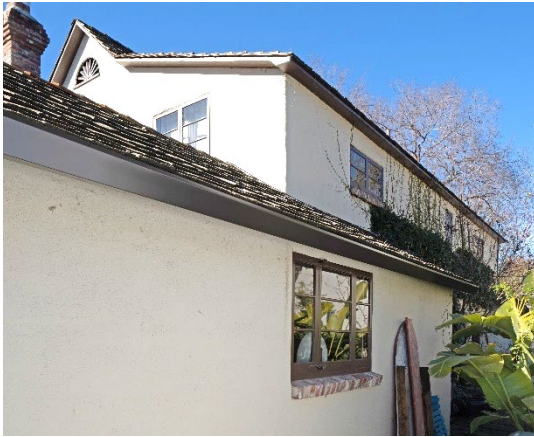
Figure 9: Looking west toward the northeast façade from the rear of the property.
