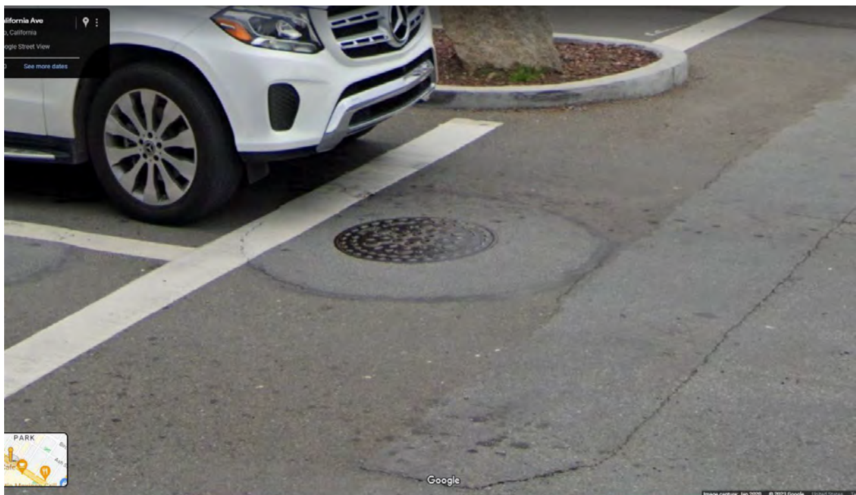
Figure 9-Google Street View Screenshot with Manhole for 16" Valve
