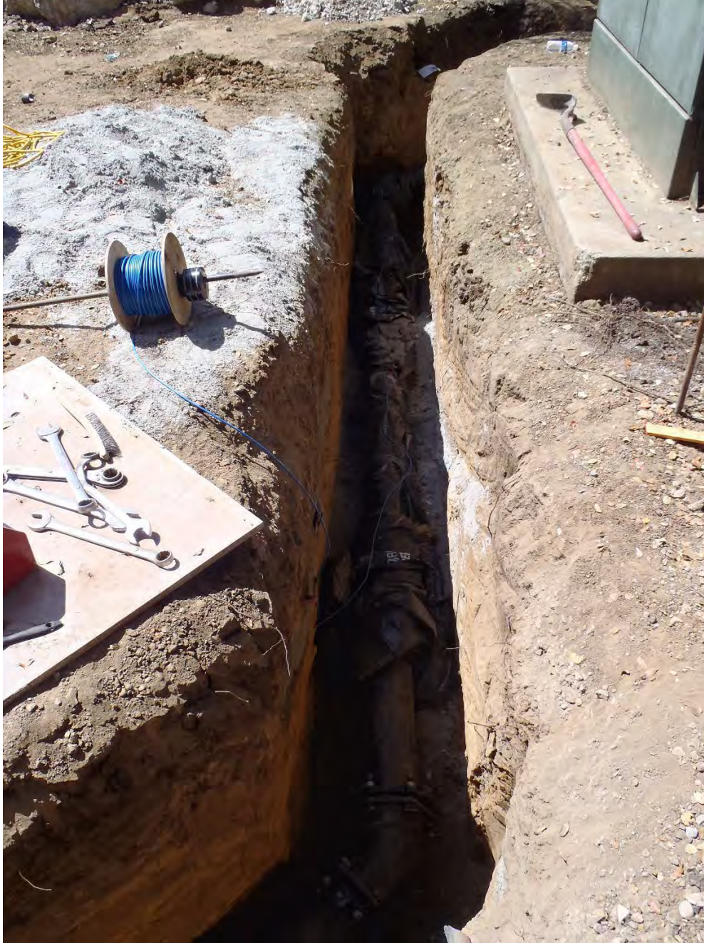
Figure 5-DIP Piping Past the Coupling to Show Depth
