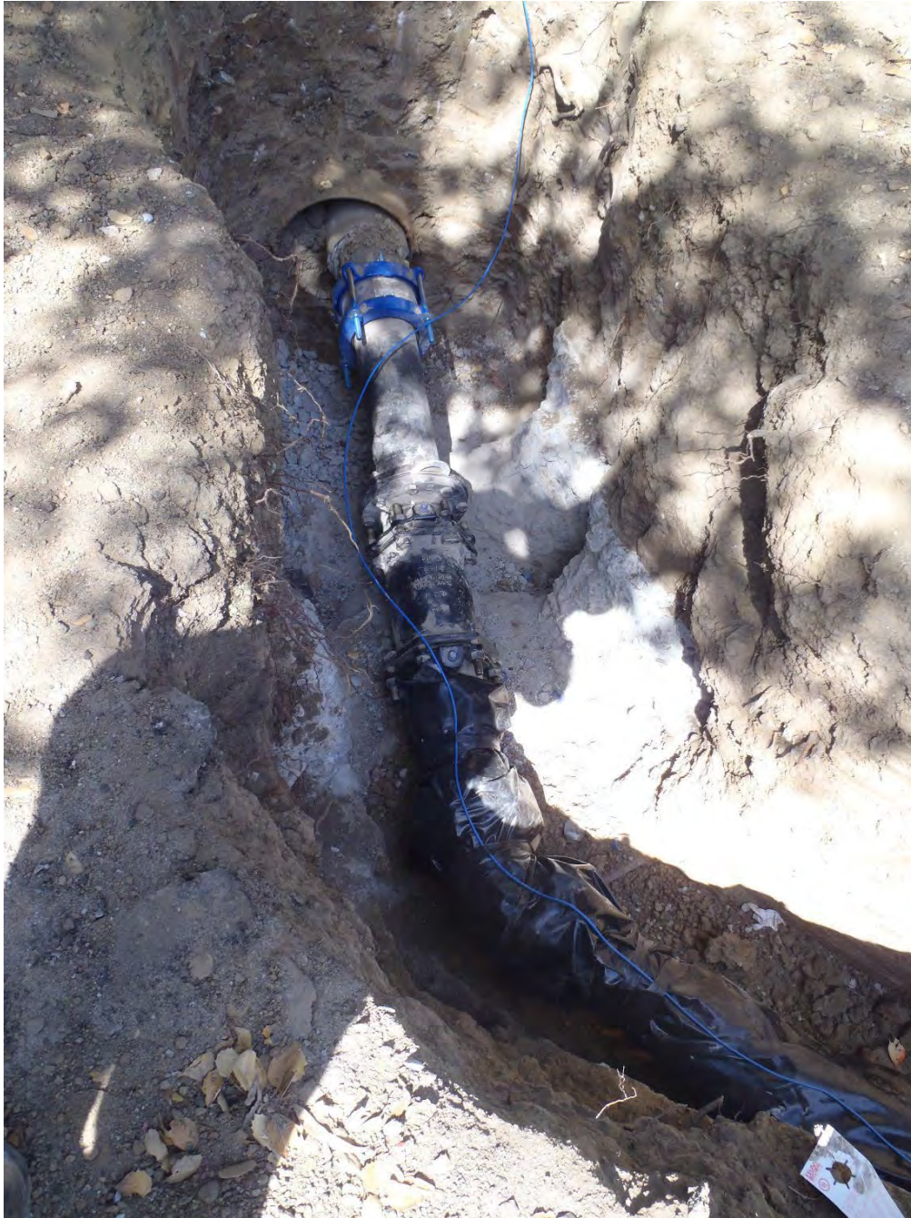
Figure 4-DIP Piping Past the Coupling
