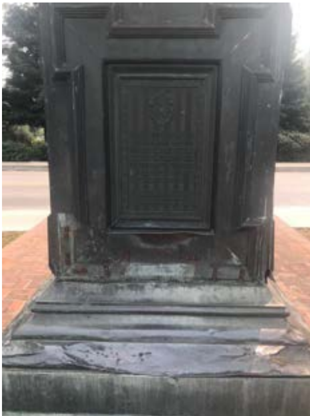
Undated crime scene photograph, prior to construction of enclosure. Damage on side facing VMB.
