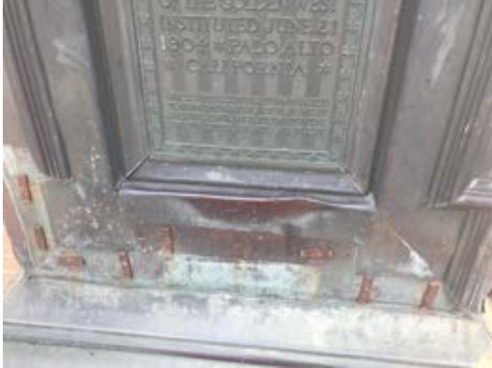
Detail of damage to copper trim
