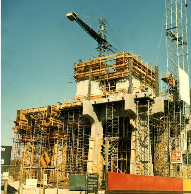
Figure 67. Construction of the Palo Alto Office Center tower base, circa 1965. Source: Palo Alto Historical Association.
