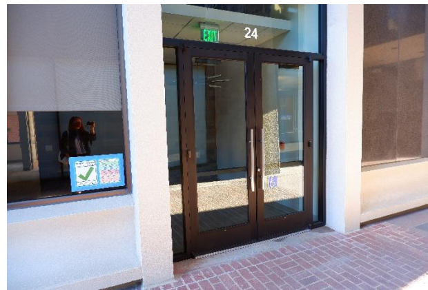
Figure 23. Non-original doors at the fifth bay from the west on the south façade.
