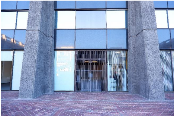
Figure 9. Metal gate at the center of the west façade, accessing a mechanical area.
