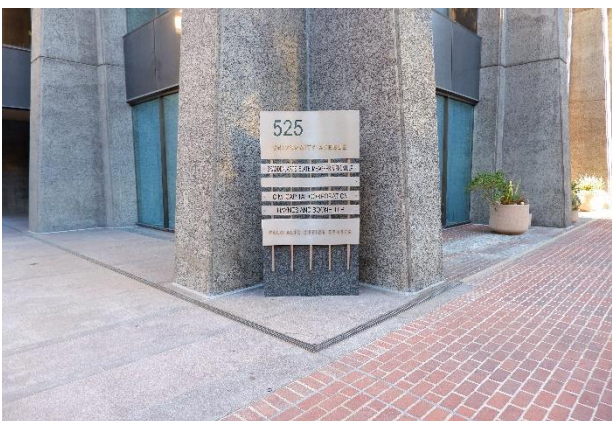
Figure 32. Original brick paving (right) and replacement granite paving (left), with free-standing sign at southeast corner of the Office Tower.
