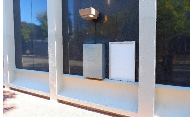
Figure 29. Former ATM location at the fourth bay from the east (right) on the south façade.
