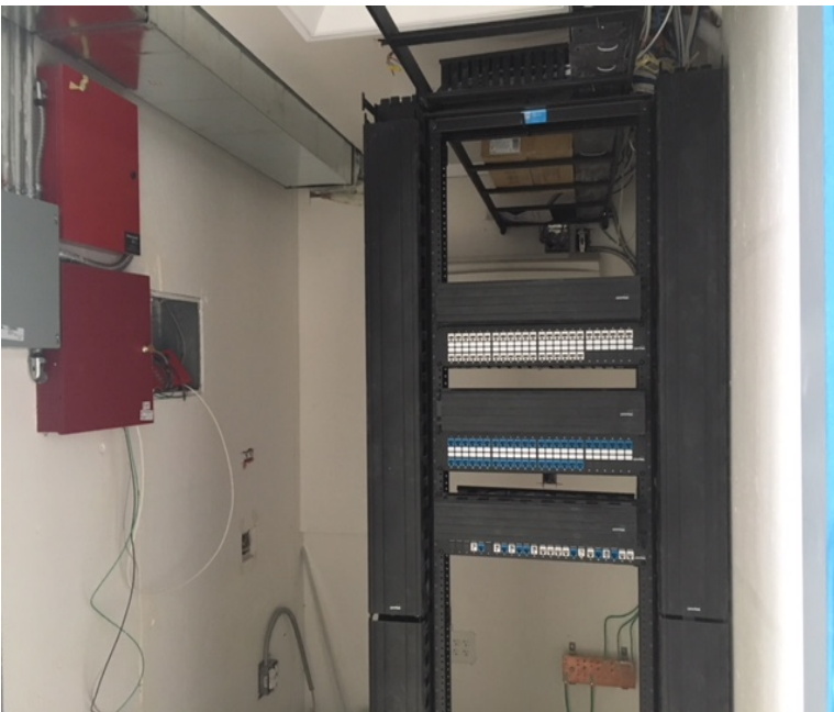
Low Voltage termination at IT rack.
