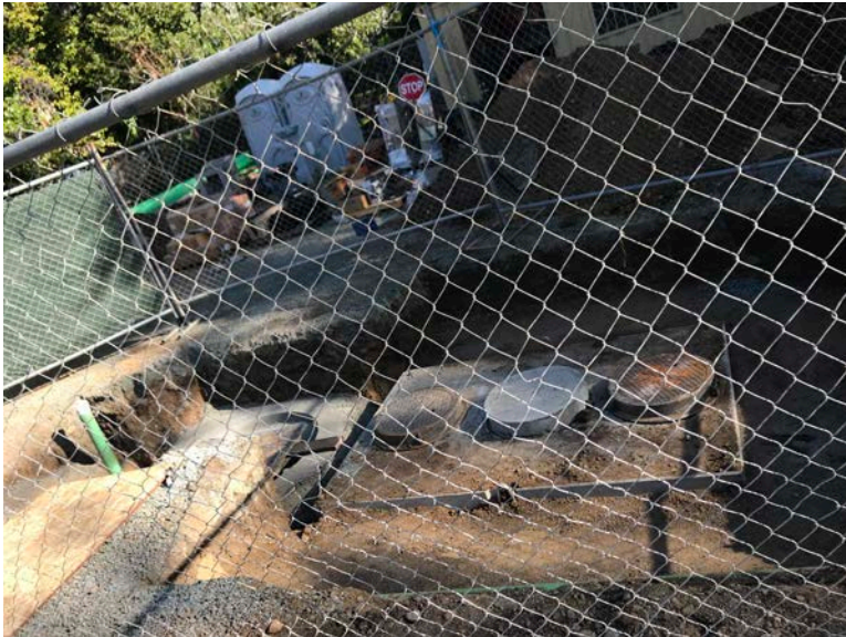
New Sand-Oil Separator installed.
