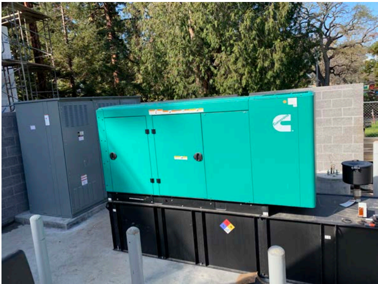
Switchgear and Generator installed onsite.
