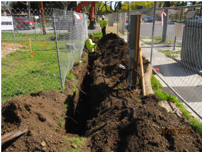
Temporary power meter installed onsite.
