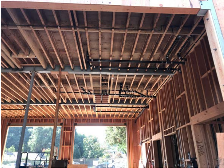
Interior plumbing in Apparatus Bay.
