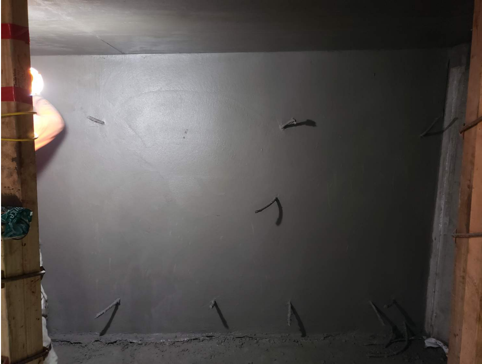
Shotcrete wall being finished. Grout injection tubes for waterproofing system shown in photo.
