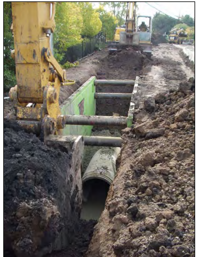
Gailen/Bibbits storm drain pipeline
