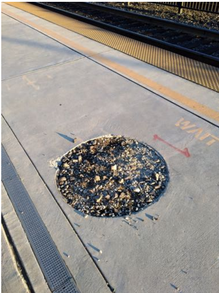
Figure 9, Misdilled pole foundation hole, in California Ave station northbound platform.
