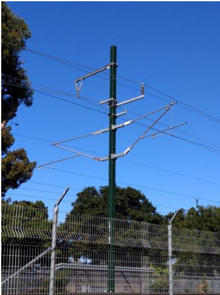
Figure 10, A standard City marine green pole, just north of the University Ave station.
