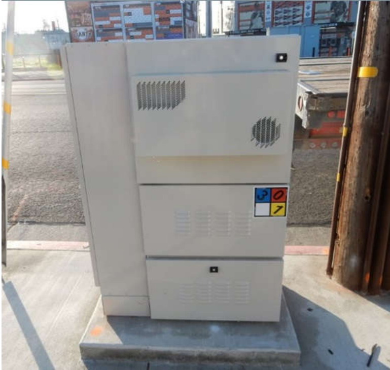
Ground mounted emergency battery cabinet without wrap.
