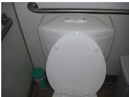
A dual-flush, low-flow toilet was installed in the building.
