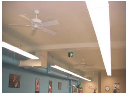
Energy efficient fluorescent lighting was installed to reduce costs and brighten the gym space
