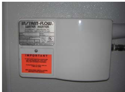
An instant water heater was installed in the bathroom
